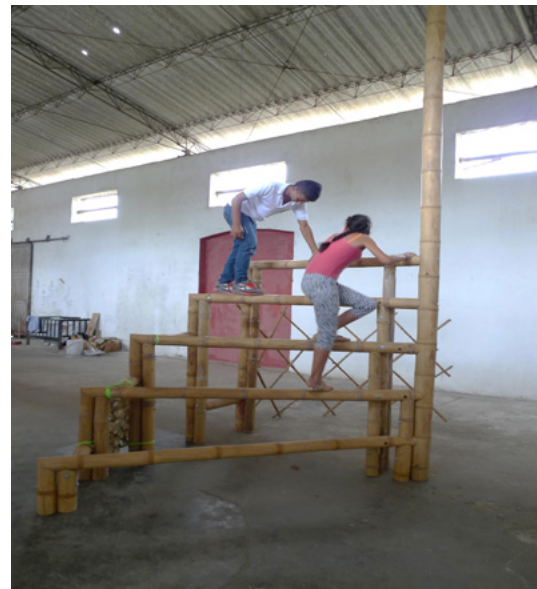
Figure 5. Bamboo structure for seating and playing- under construction and in use by local kids. (Estudio SPN).
